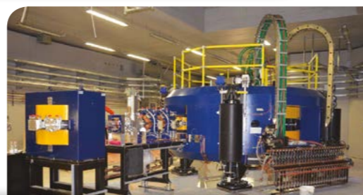
Installation of Best 70 MeV Cyclotron at Italian National Laboratories (INFN), Legnaro, IT
