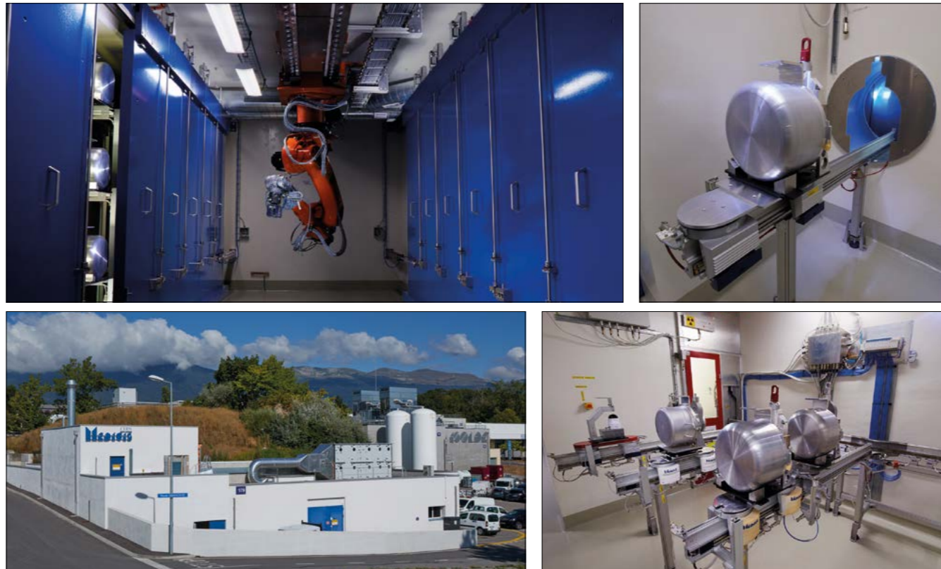
Clockwise from top left: Storage shelves for ISOLDE and CERN-MEDICIS targets after their operation, showing the robot for remote handling. A “fresh” target unit stands on the CERN-MEDICIS supply point, ready for the robot pick-up and transportation to the irradiation point. A rail conveyor system end-station for target transportation, showing the inspection camera and two modern target units. The MEDICIS building at CERN, next to ISOLDE. (Image credits: Yury Gavrikov.)
