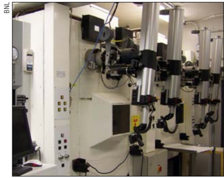
Two of the hot cells used for radioisotope processing at BNL to protect workers from high radiation levels while performing chemical separation.
